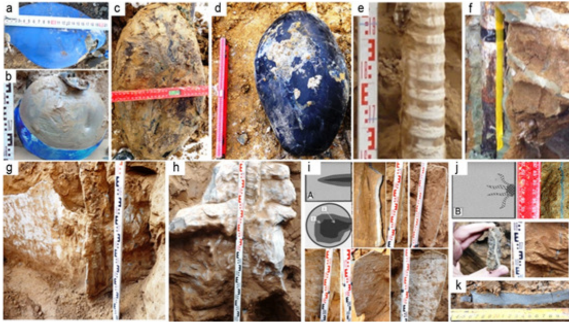
Figure 2 Geometric features of the proposed piles: a, b - controlled broadenings of 10-20 liters; c, d - controlled broadening of 30-40 liters; e - increase in diameter of the pile stem; f - formation of hydraulic fractures; g, h - the nature of the spread of hydraulic fractures during the first and repeated injection of the solution, respectively; i,j- the types of fracture textures A and B, respectively; k - horizontal hydraulic fractures
