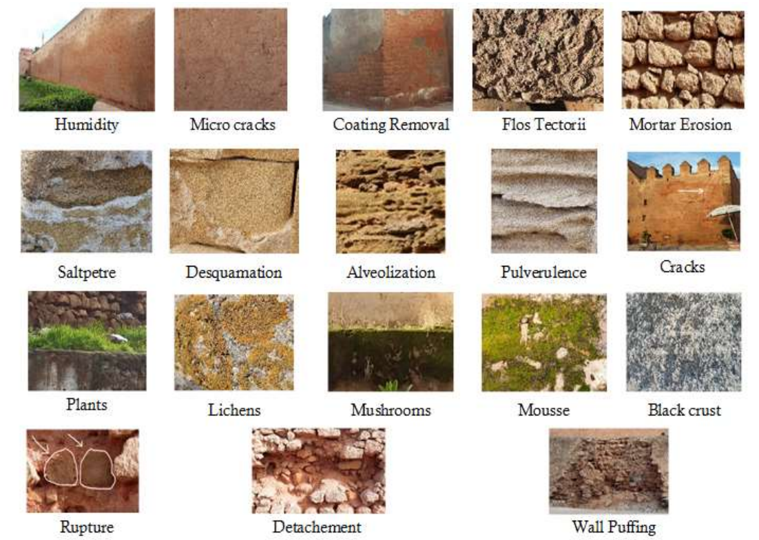
Figure 3 Examples of forms of alteration on walls.
